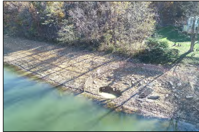
Figure 3. Sinkhole Development Along Shoreline
