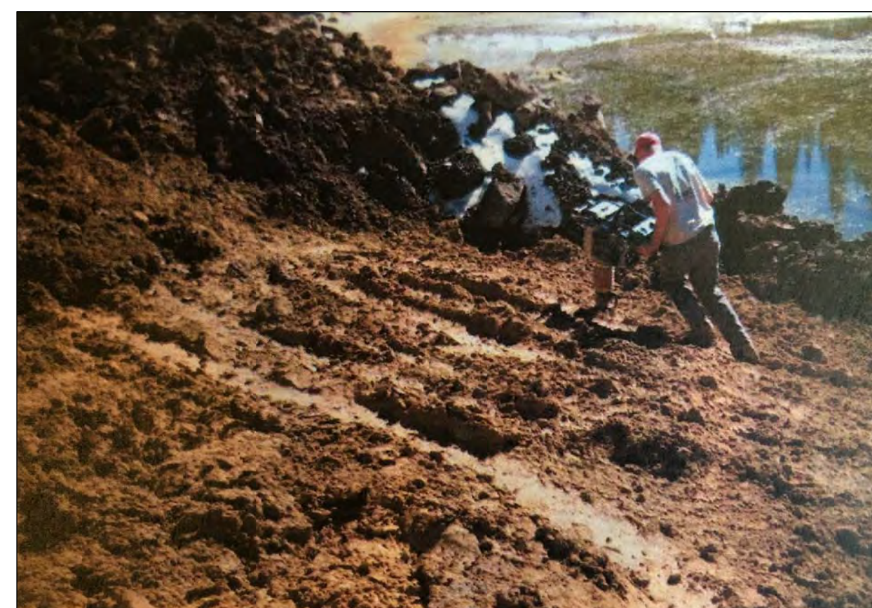
STEP 5: Compact backfill to 95% ASTM D698. Minimum 12-inch cover required over liner system.
