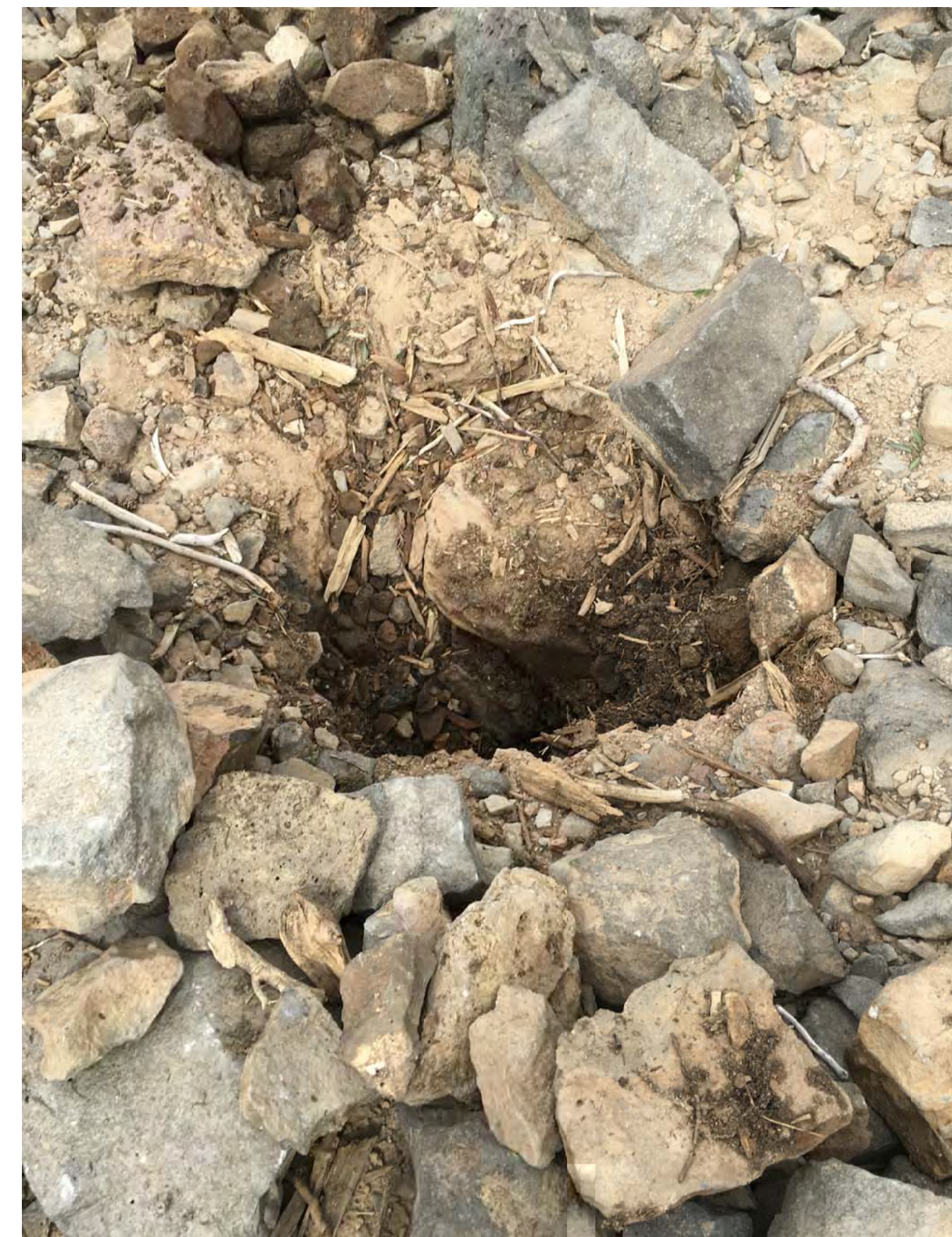
NEW SEEP HOLE
